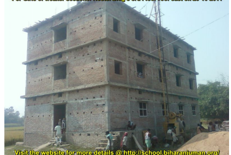
RAHBAR-e-Banaat School and Madrasa, for holistic education & guidance For Girls of weaker sections: Hostel Bldg's 3rd Floor roof cast on 29-10-2011
